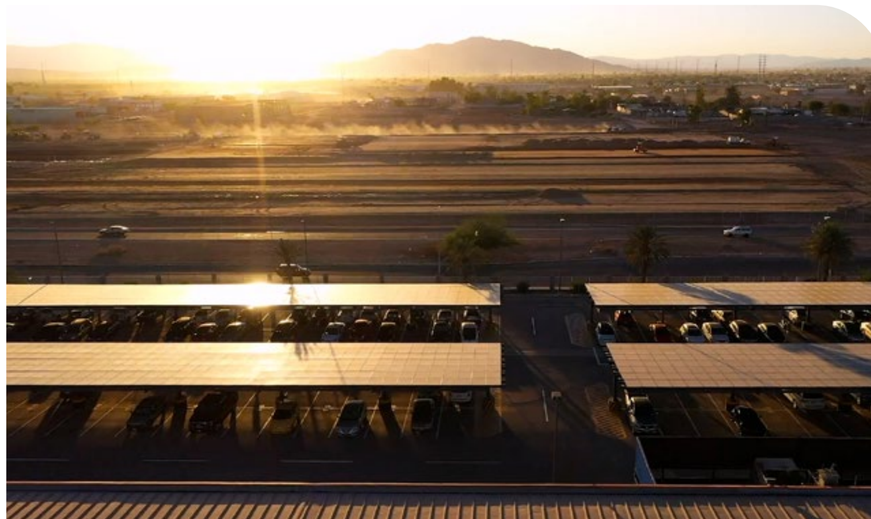
Carport solar in Mexicali, Mexico facility
